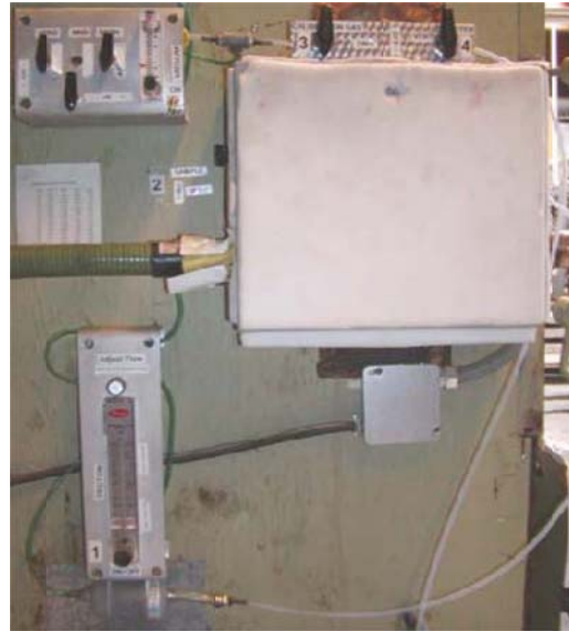
Figure 9. Schematic of heated filter box with air dilution system, heated sample line, and analyzer (left). Sample enters heated box from back of drawing (box is attached to kiln). Photo (right) of heated box (large white box), calibration gases in (valves upper left), dilution air valve (lower left), line to analyzer (green line at left), and valve for alternate air intake (top right).
