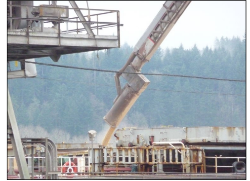
Ship loading spout. The square "box" is the deadbox and the spring loaded gate is located approximately halfway from the deadbox to the end of the spout.
