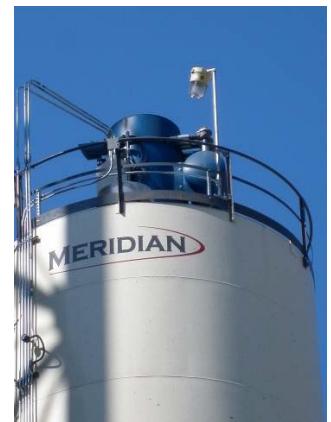
Bin Vent Filter DC-23
