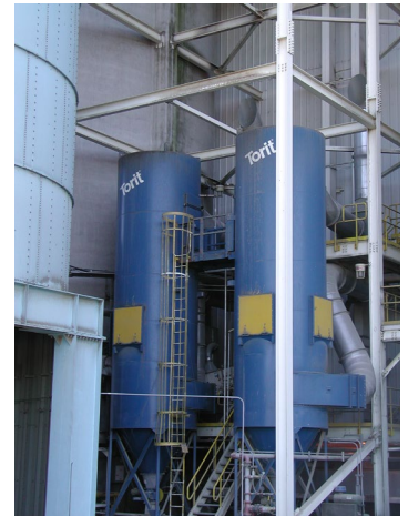
Baghouses DC-15 (left) and DC-17 (right)
