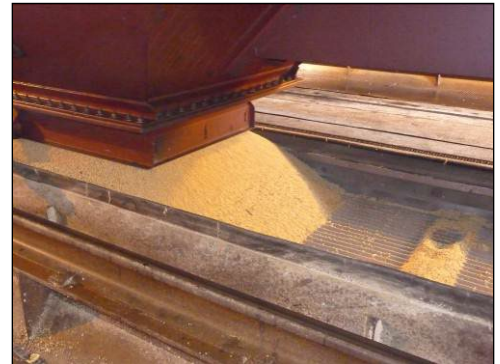
Railcar receiving choke flow
