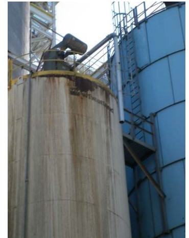
Bin Vent Filter DC-19
