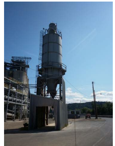
Bin Vent Filter DC-13
