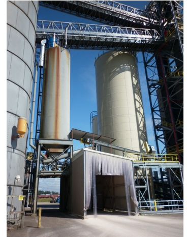
Bin Vent Filter DC-12 (top left)
