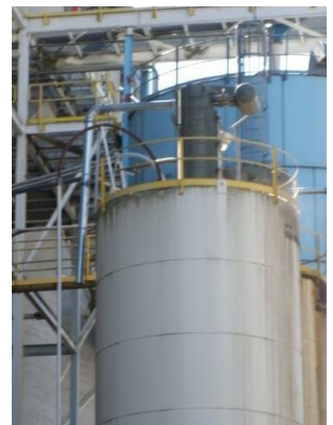
Bin Vent Filter DC-18
